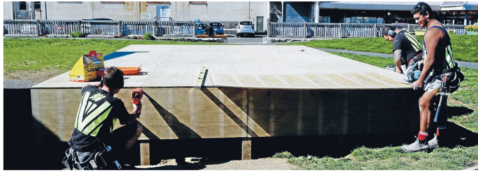
Steven Harvey, Casey Cumming and Metua Aerenga, three of the many builders from several companies that helped build the stage.
